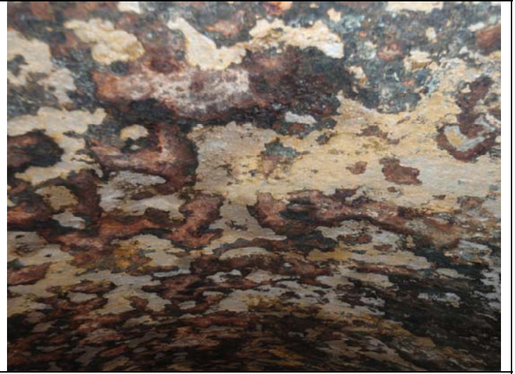
Scaling and general corrosion on upper shell
