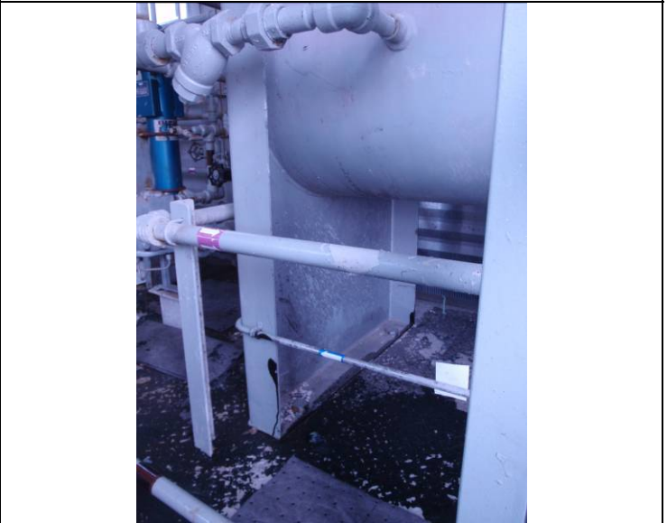
Bolted to skid floor
