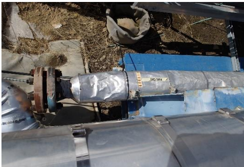
Figure 7: Blinded gas inlet to separator
