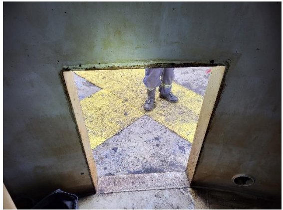
Manway internal overview
