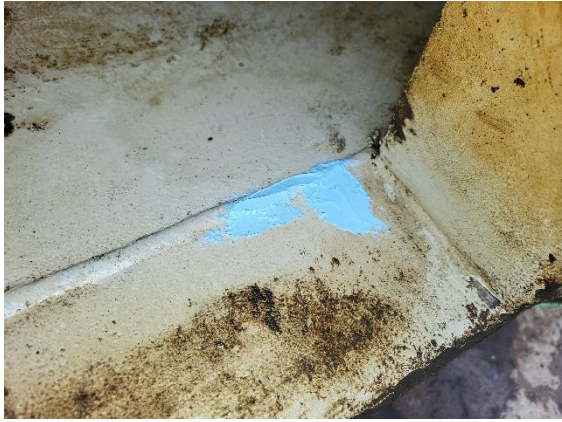
Epoxy patch area
