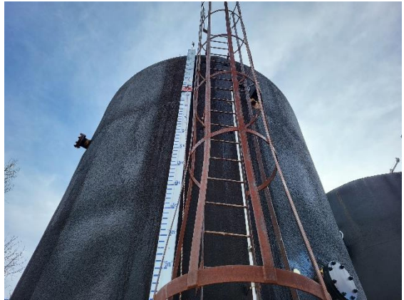
Ladder - level gauge overview
