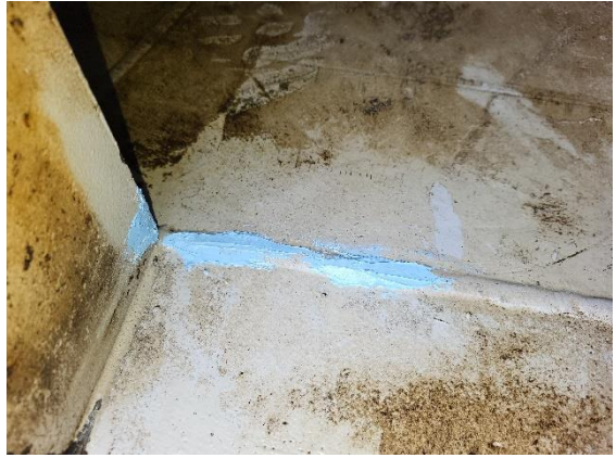
Epoxy patch area
