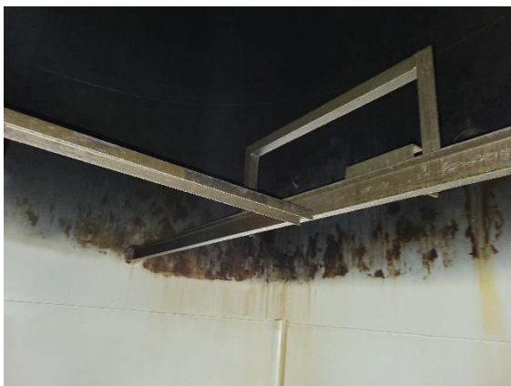
Heating tube support - tube permanently removed
