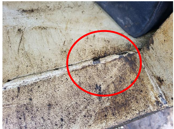
Coating chipped on manway weld
