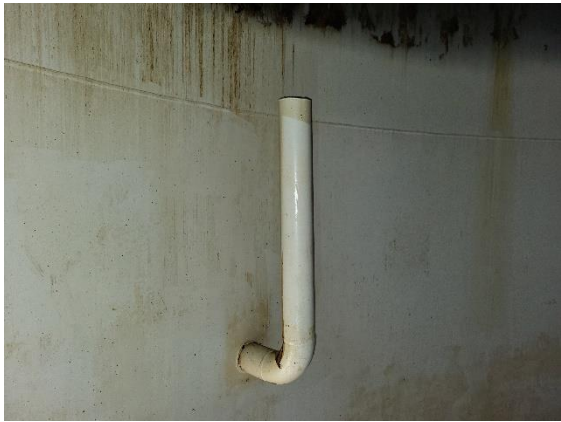
Internal piping overview
