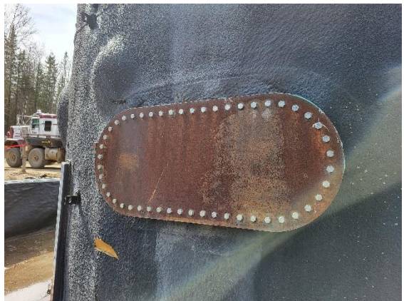
Heating tube covering
