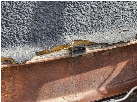
base to skid connection
