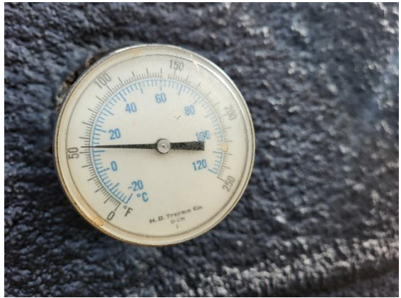
Temperature gauge overview
