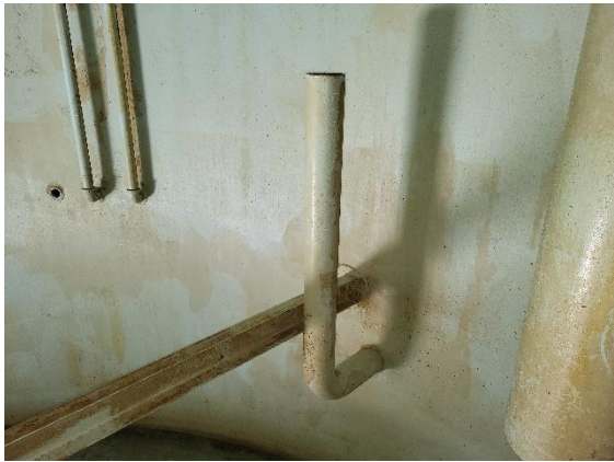
Internal piping overview
