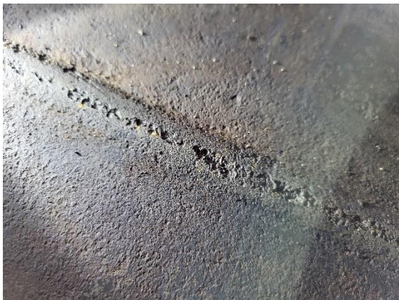
Floor weld cap pitting
