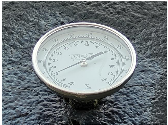
Temperature gauge overview
