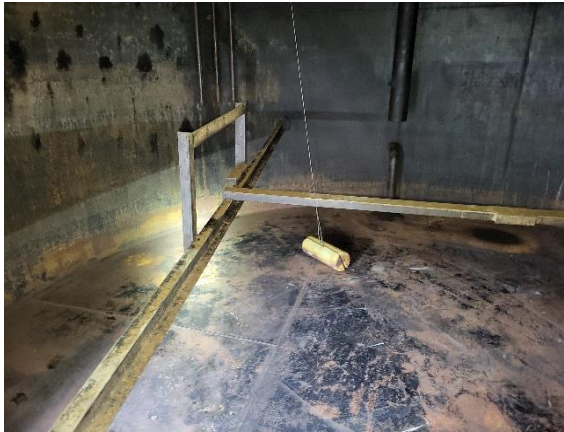
Heating tube support - tube permanently removed
