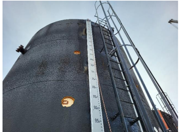
Ladder - level gauge overview
