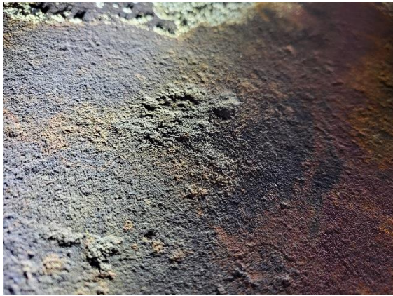
Floor general corrosion .020 inch
