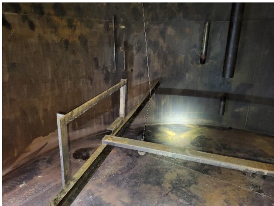
Heating tube support - tube permanently removed
