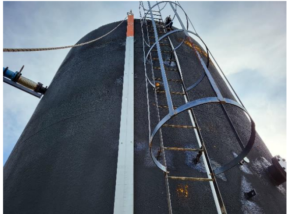
Ladder - level gauge overview
