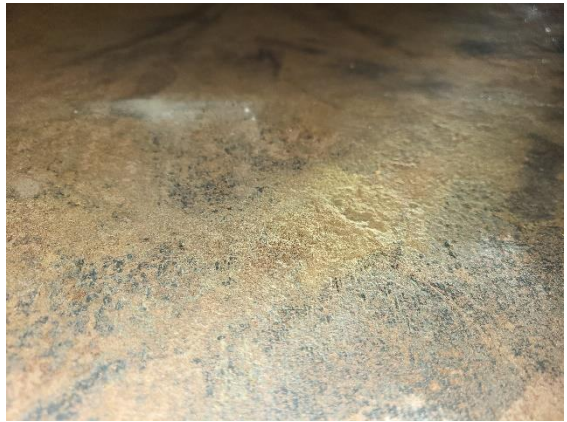
Floor general corrosion .010 inch
