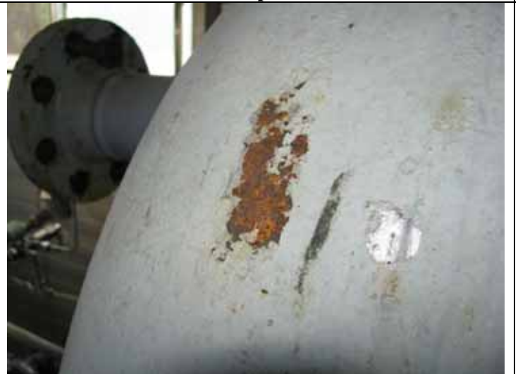
Minor pitting in areas of paint failure on shell and head.
