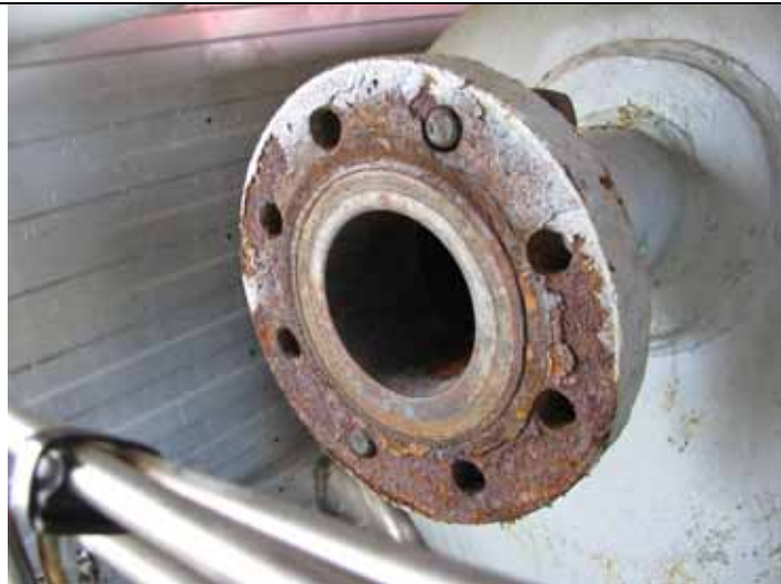
Pitting and corrosion to flange face.
