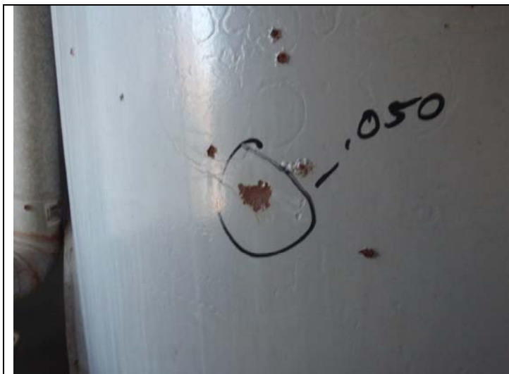
External pitting on lower shell
