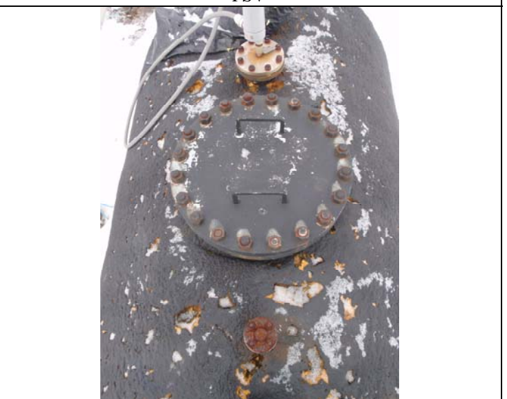
Multiple tears in insulation along top shell
