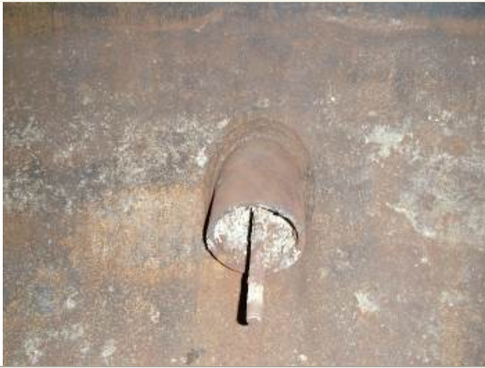
100% Consumed anode at the oil end of Treater.
