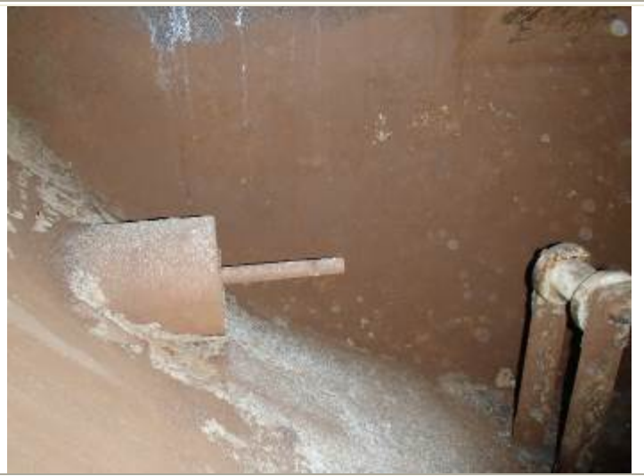
100% Consumed anode at the emulsion end of Treater.
