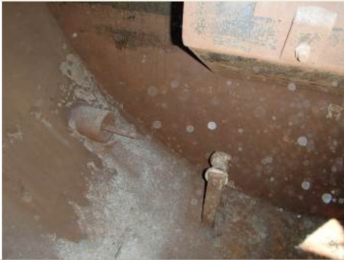
Attachment hardware intact.
