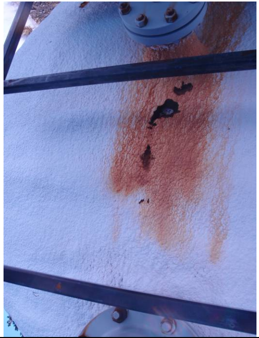
damage to insulation - inlet
