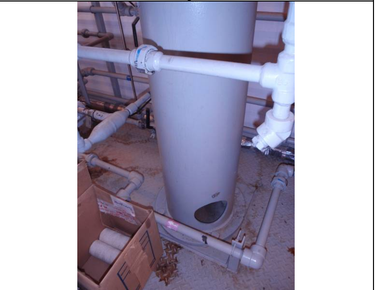
Bolted to skid floor
