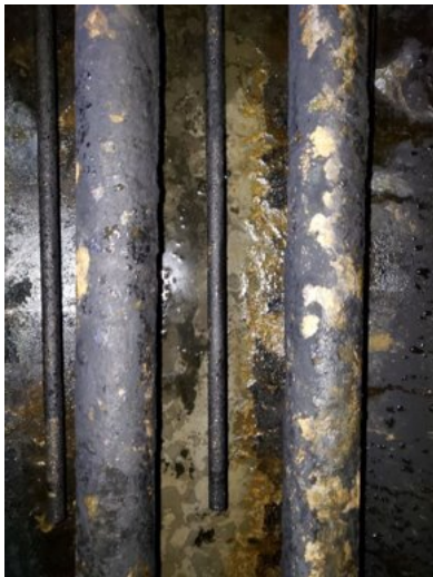
Corrosion Line Along 6:00 Below Coil
