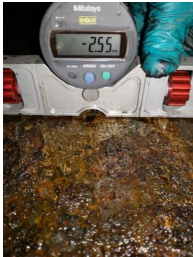
North Shell Section West Side 9:00 Pitting
