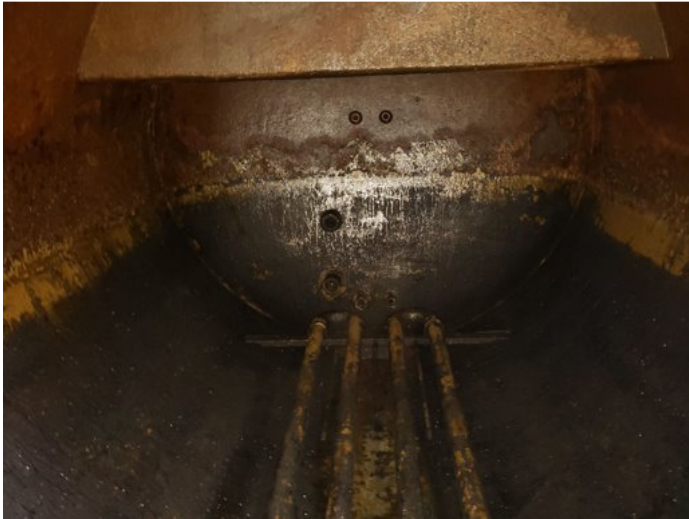
South End of Vessel Corrosion Line
