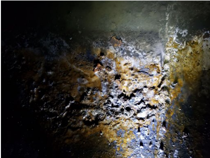
North Head to Shell 6:00 Pitting
