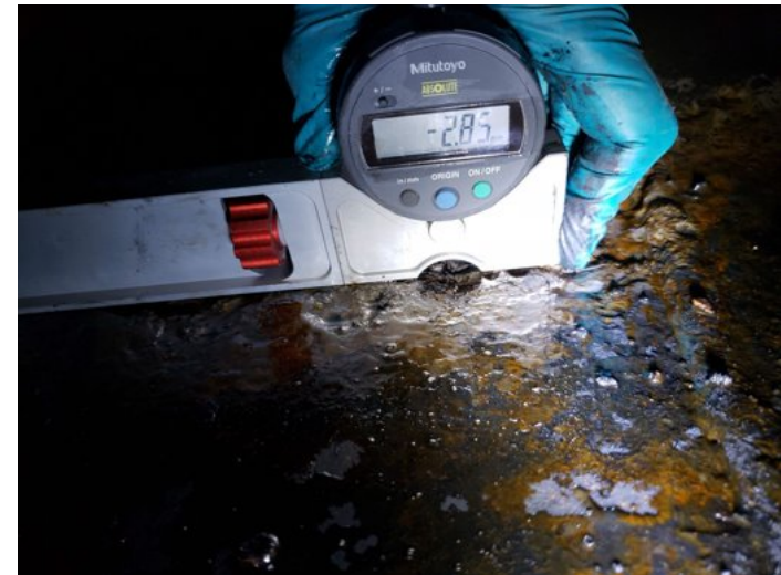
North Head to Shell 6:00 Pitting
