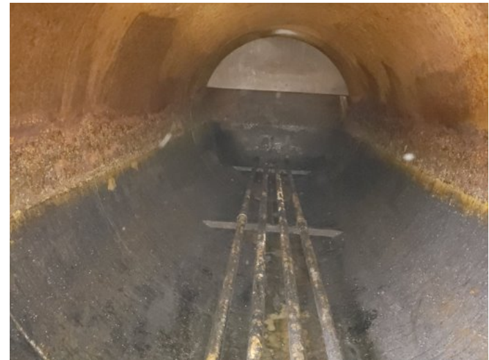
North End of Vessel Showing Fluid Corrosion Line 9:00 & 3:00
