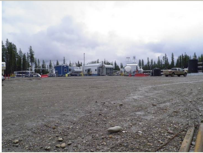
9-21- Compressor site overview.
