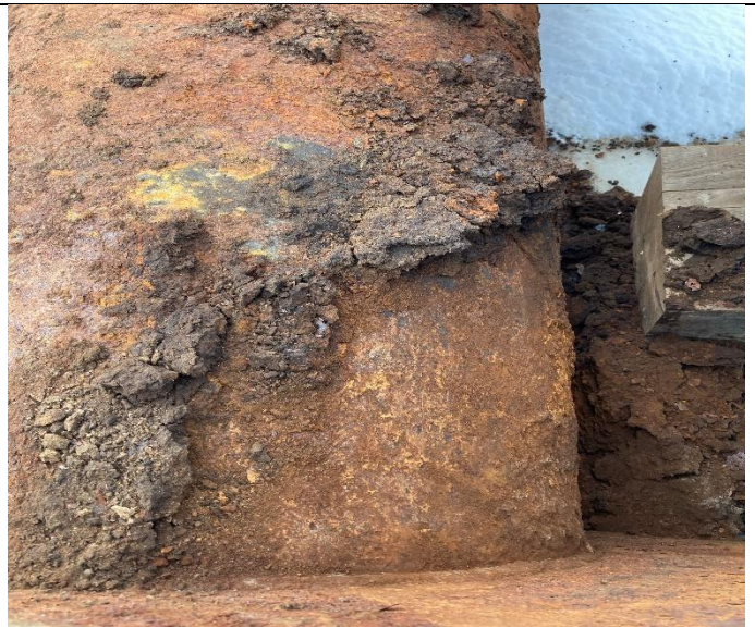
External corrosion on Firetubes due to oil and sand build up
