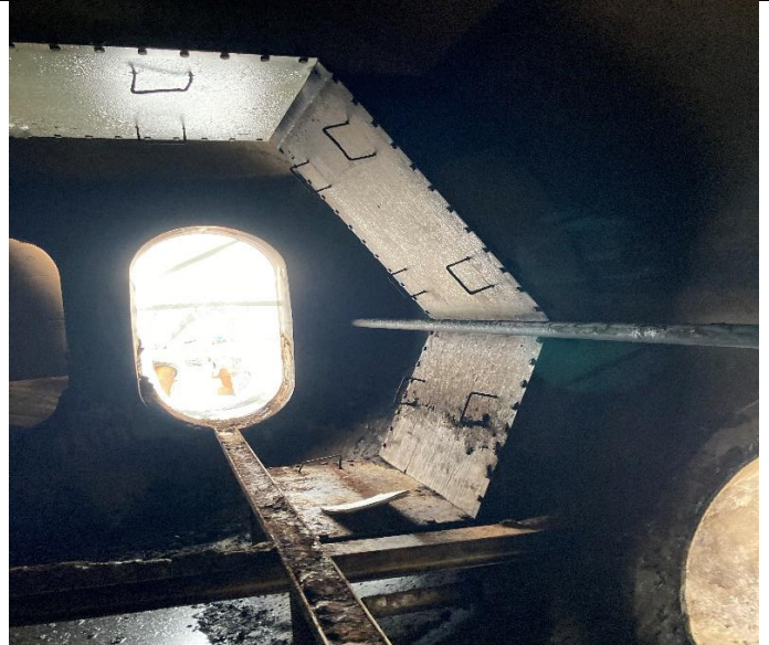
Inlet diverter prior to cleaning
