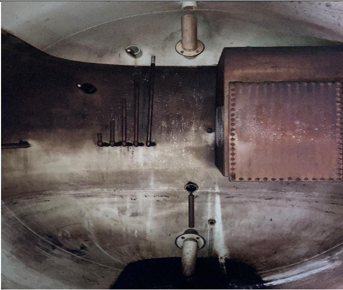
Oil end internal picture of oil box and sample connections
