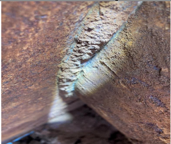
External corrosion on plate to tube weld due to oil and sand build up
