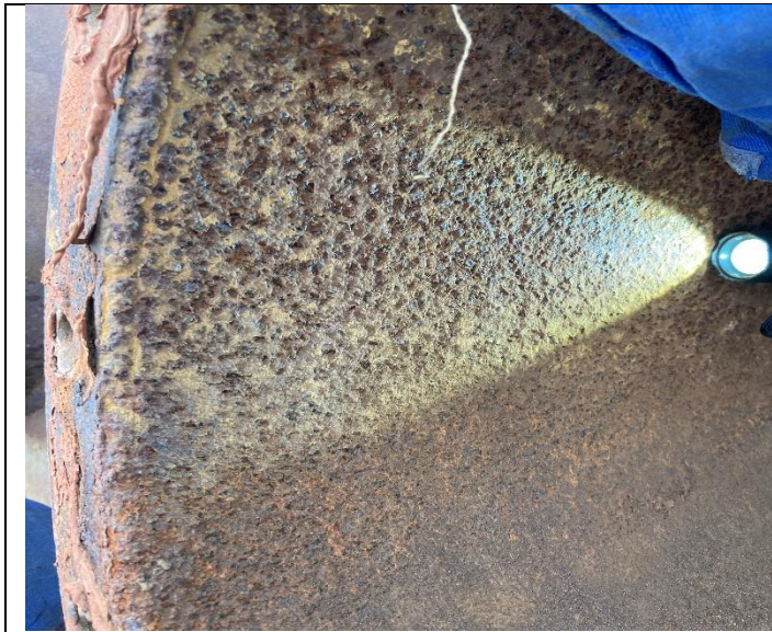
Top tube of Firetube corrosion due to rain and contaminants through stack
