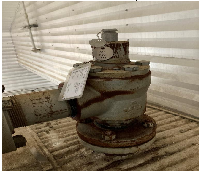
Vessel PSV installed on Nozzle N10
