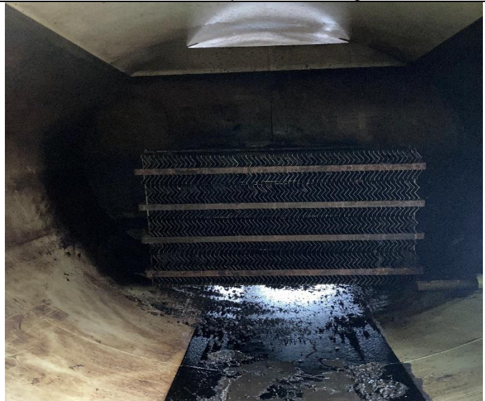
Weir and Coalescing pack prior to cleaning
