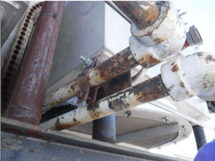
11-Loose support in contact with adjacent burner pipe
