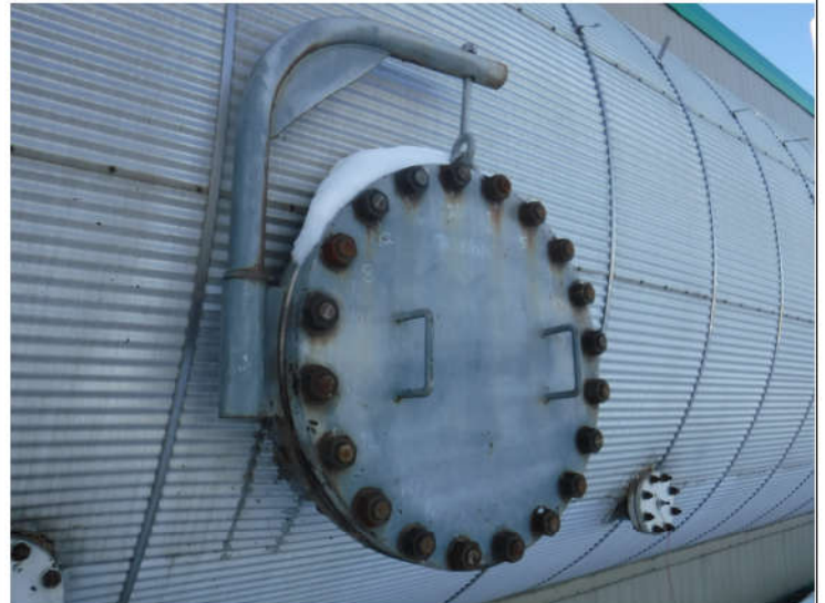
04-Corrosion on manway, nuts and bolts, no depth
