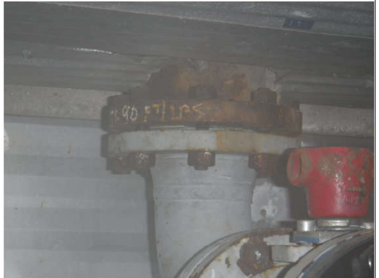
12-Significant corrosion on bottom nozzles, nuts and bolts
