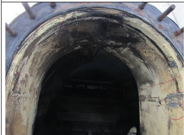
Coating damage and blistering to upper portion of fire tube nozzle left
