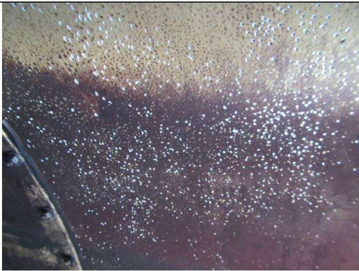
Coating blistering to inlet defuser – not pressure envelope
