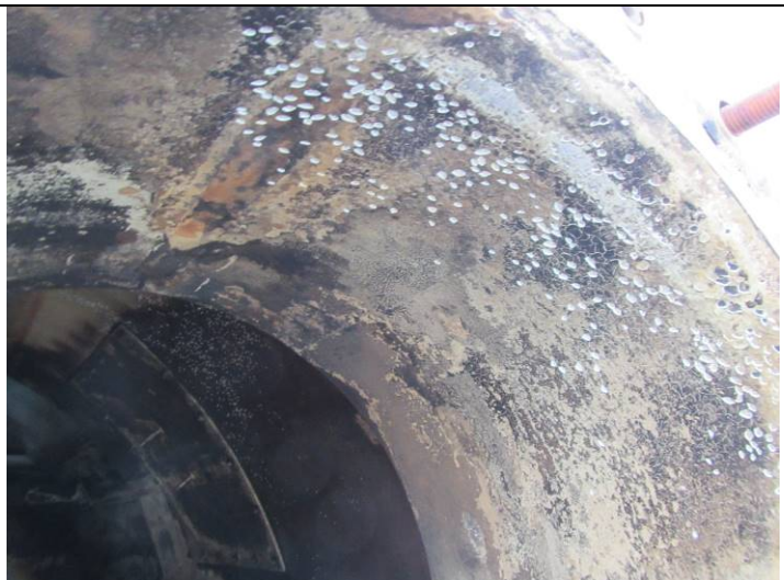
Coating damage and blistering to upper portion of fire tube nozzle right
