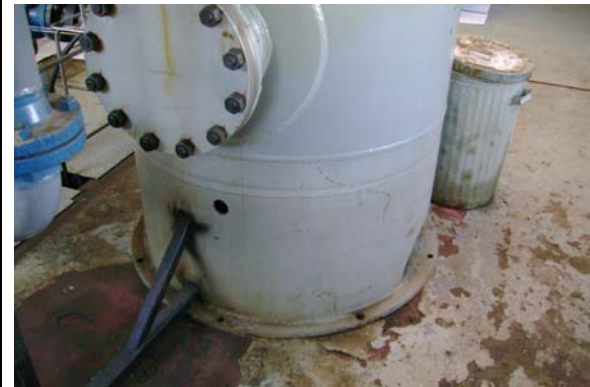
vessel skirt not anchored
