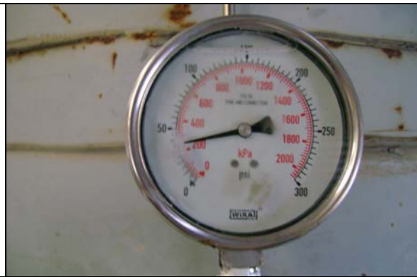
vessel pressure gauge
