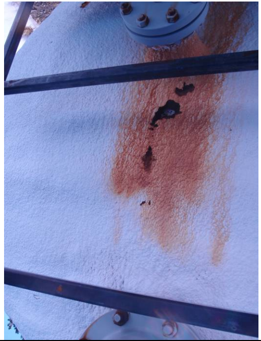
damage to insulation - inlet
