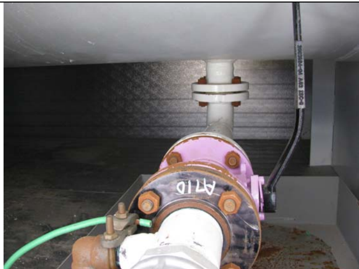
Truck-out piping is in good condition.
