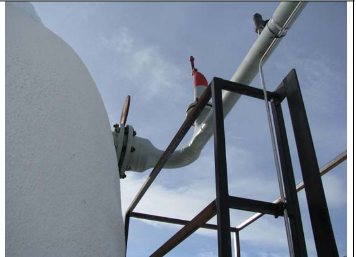
Piping is in good condition and well supported.
