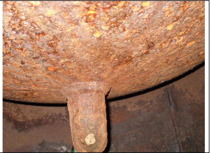
Heavy External scaling under skirt
