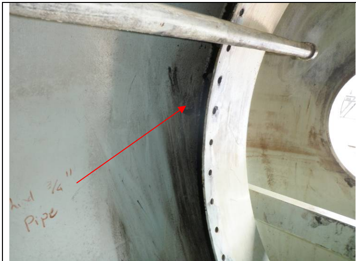
Coating failure at shell
