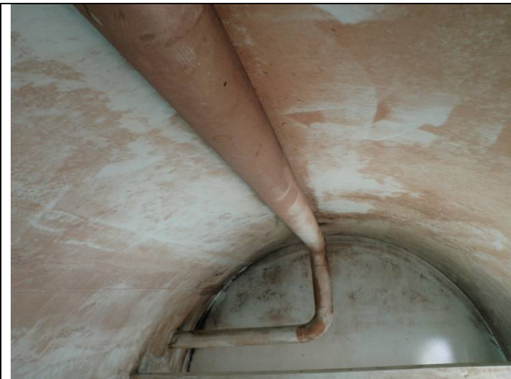
Upper shell and inlet piping
