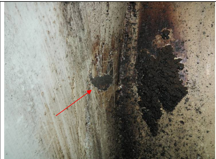
Coating Failure - surface corrosion to depth of 0.010 inch
