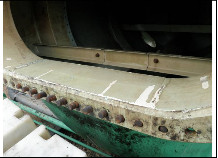
Previous coating repairs
