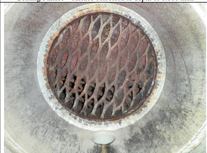
Demister pad - dirty and corroded
