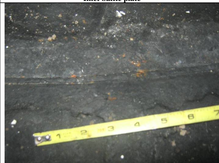
Corrosion at north head to shell weld
