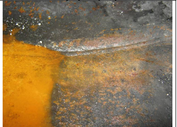
South head weld – minimal corrosion
