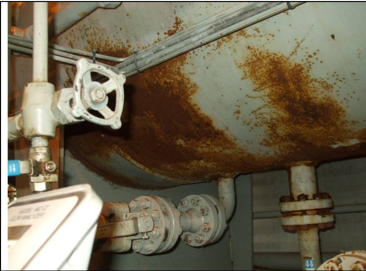
External corrosion to 30% of shell
