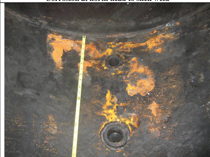
Water side corrosion at weir plate to max depth of 0.150 inch
