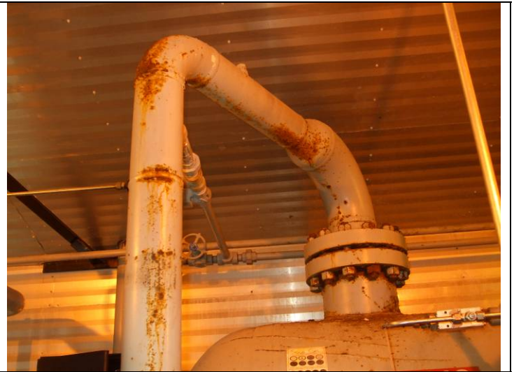
External corrosion to 30% of the piping surfaces
