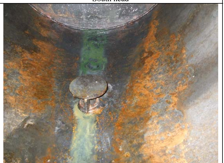
Lower shell pitting to 0.120"
