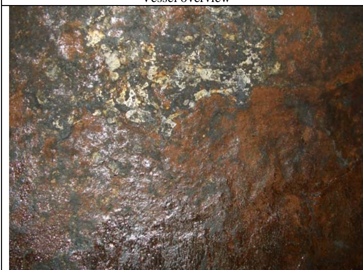
Lower shell pitting to 0.120"
