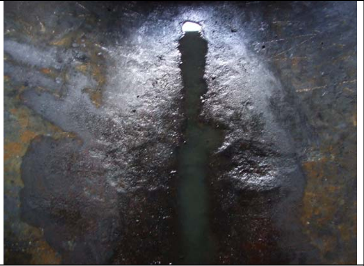
Lower shell pitting to 0.120" @ manway
