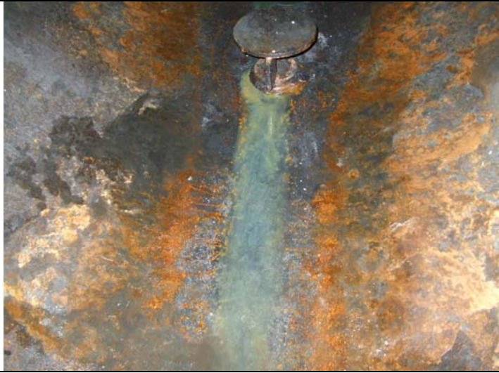
Lower shell pitting to 0.120"
