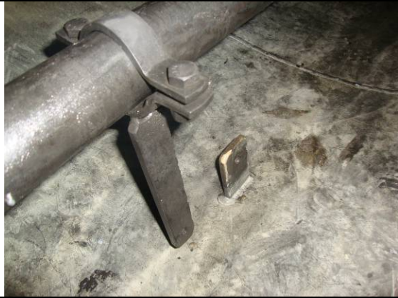
Missing bolt on pipe support
