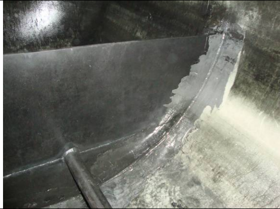
Weir and pipe attachment
