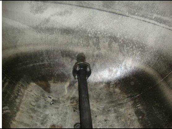
Vessel heat and pipe nozzle attachment
