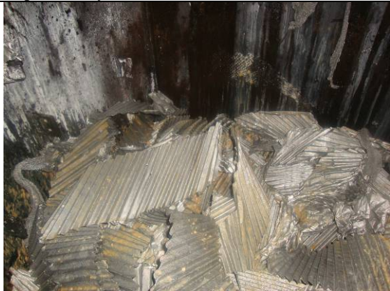
Damaged packing under top man way
