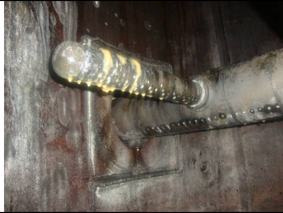
Piping attachment to shell
