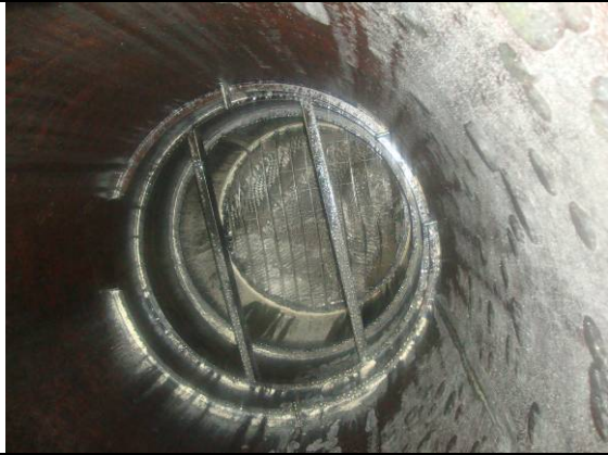
View up in the vessel at packing
