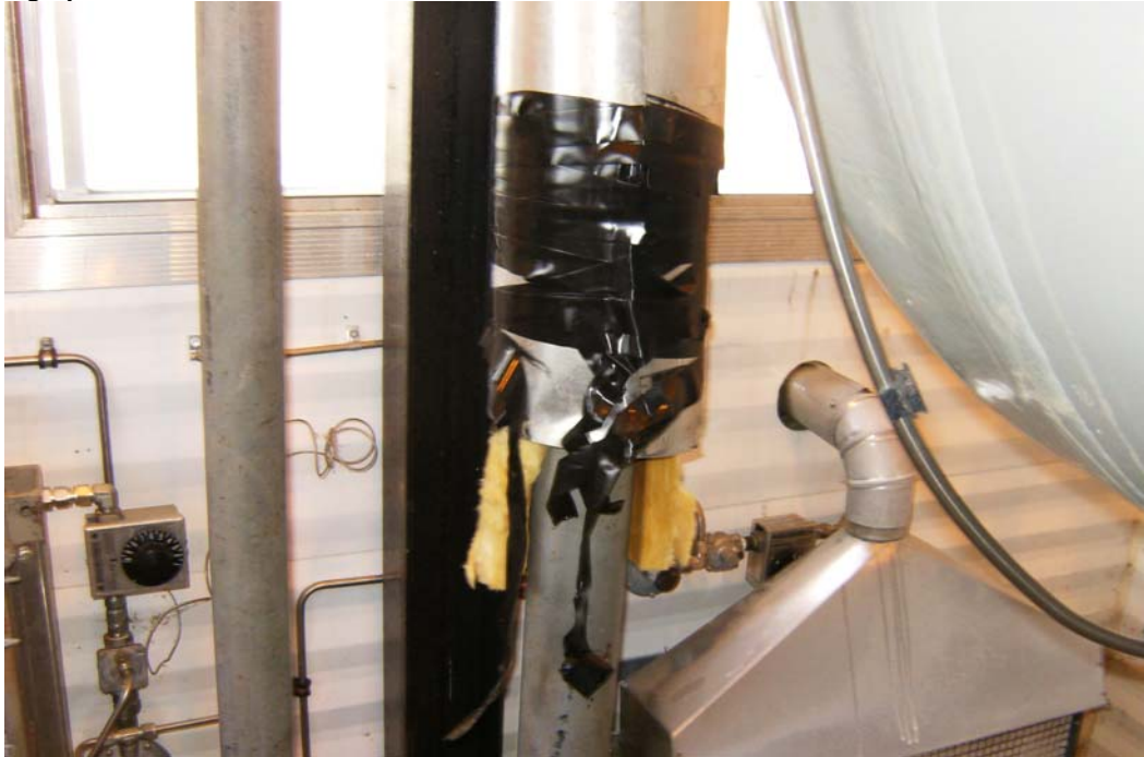
Figure 5_Insulation Damage to Drain Piping_13May09
