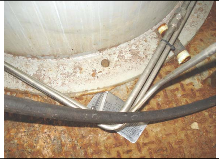
Skirt weld, note not welded.
