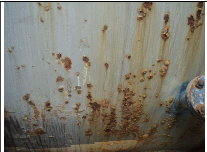
Spotting external corrosion on shell
