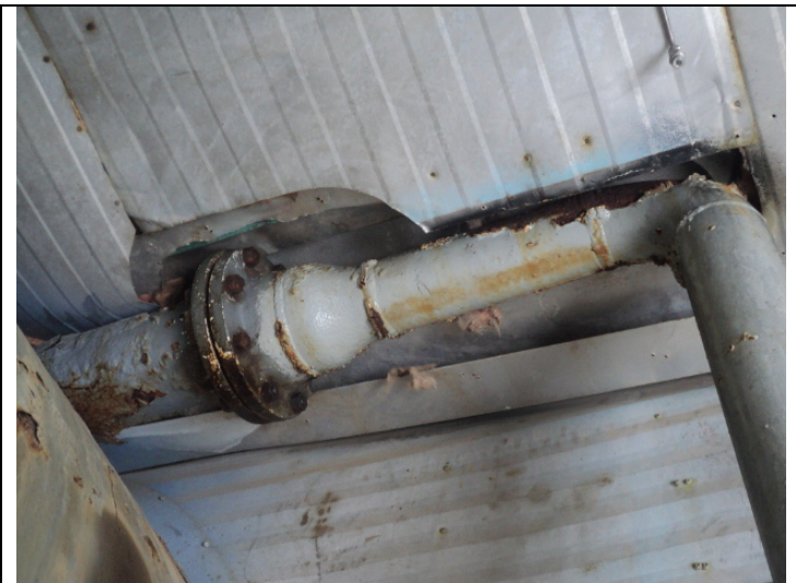
General Overview of Inlet piping
