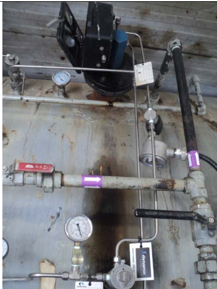
Evidence of external staining due to seepage
