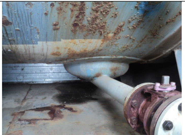
Spotting external corrosion on lower shell and boot
