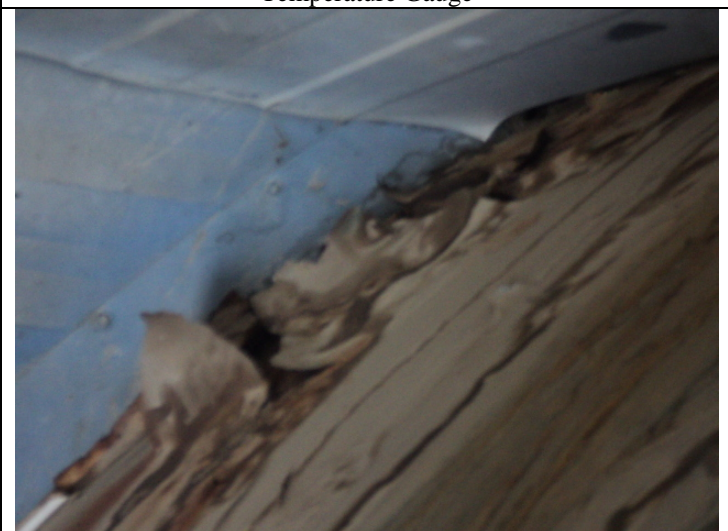
Paint peeling at 12 O'clock
