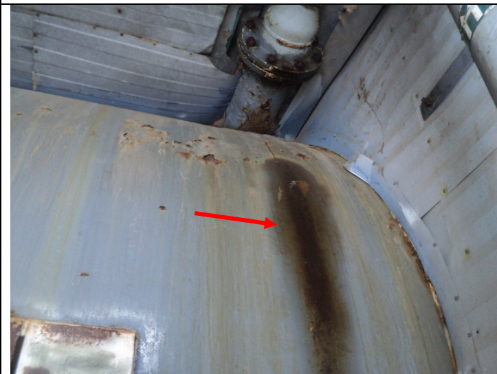
Evidence of external staining due to seepage
