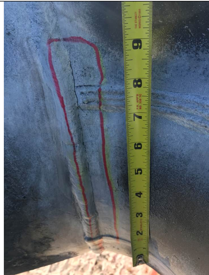
Overview of crack number 1 on circ weld
