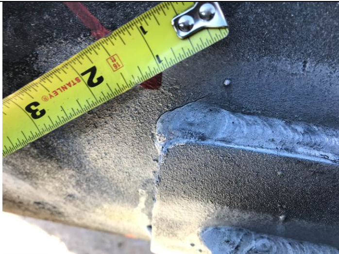
Overview of crack number 3 on anchor support
