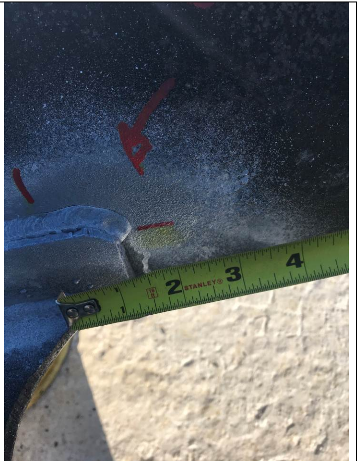
Overview of crack number 2 on anchor support
