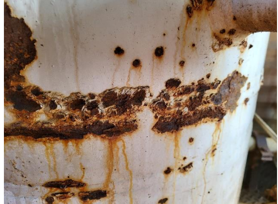
Shell paint condition
