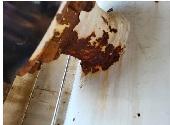
Nozzle paint condition
