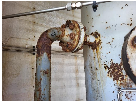
Inlet piping overview
