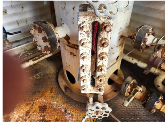
Liquid level gauge overview
