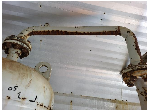
Gas out piping overview
