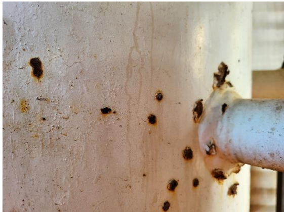
Shell paint condition
