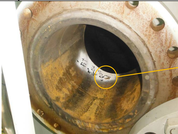
North 14 inch manway - Isolated pit 5/8 inch dia. x 0.110 inch depth
